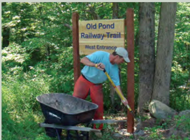
FBC Board member Randy Ewins installs the new sign at the Old Pond Railway Trail.
